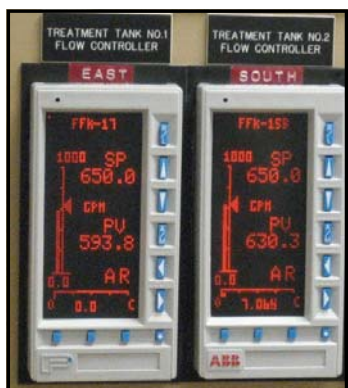
Flow Control Meters
